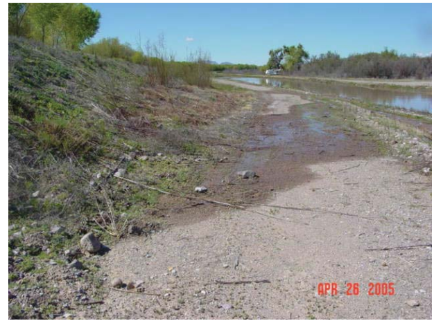
Figure 5. Socorro Levee conditions
